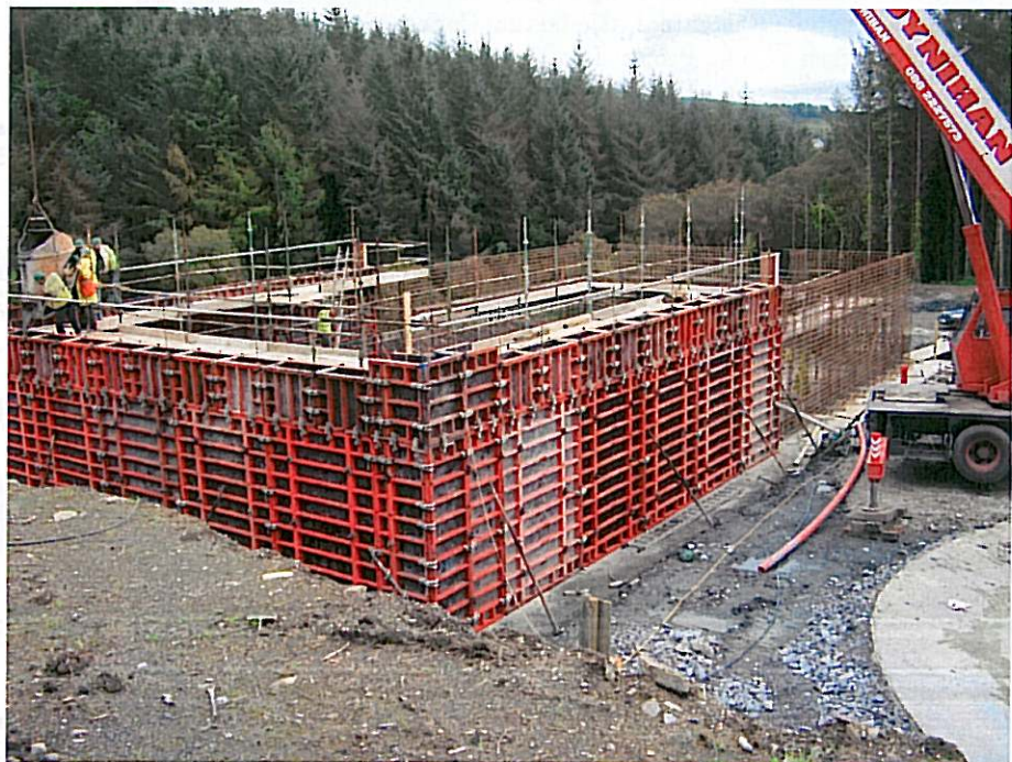
Photograph showing construction of one of the reinforced concrete treatment tanks at the site of the Wastewater Treatment Plant at Beech.
